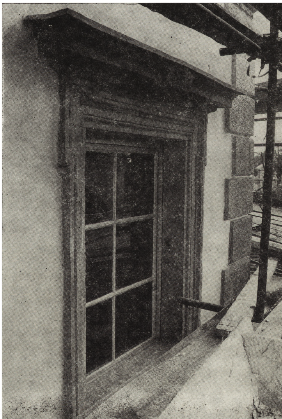
4. A stone shutter in the north-east tower: A – condition before conservation, B – condition after conservation
