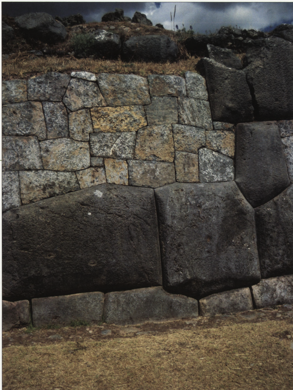
3. Ubytki w murach Sacsayhuaman. 3. Missing fragments of walls in Sacsayhuaman.
