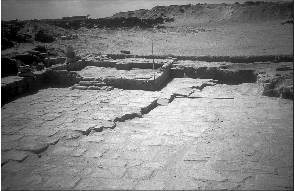
Fig. 18. Main square. Southwestern room with base (sanctuary ?); note the seismic-related dislocation of the flagstones running across the square (Photo W.A. Daszewski)
