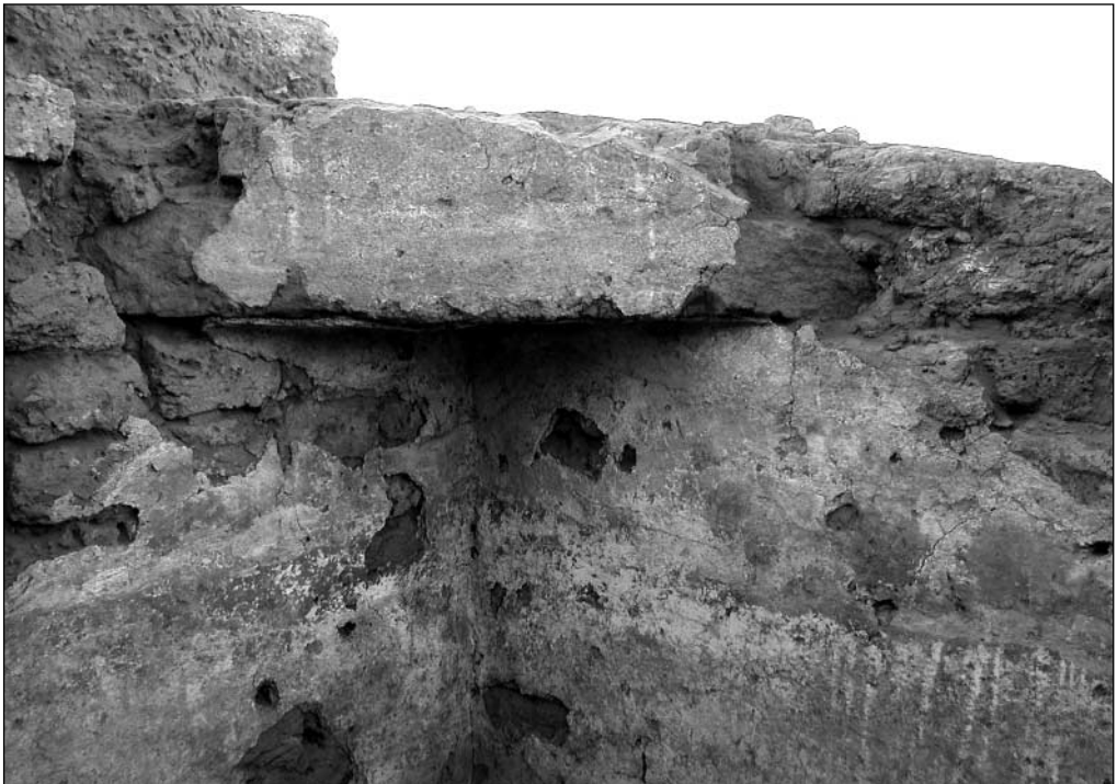
Fig. 9. Cruciform Building (B.III.1). Pendentive of the dome in the outer northeastern corner of the structure (Photo W. Godleuski)
