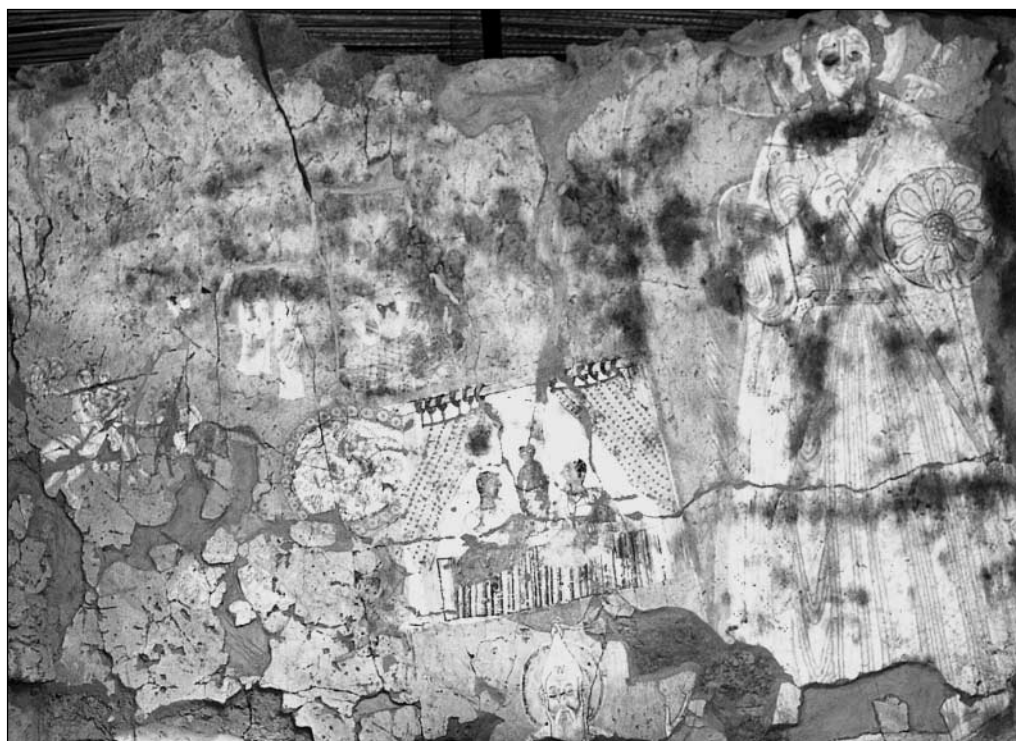
Fig. 11. Full view of the preserved murals on the south wall of room 6 in the SW Annex (Photo H. Pietras)
