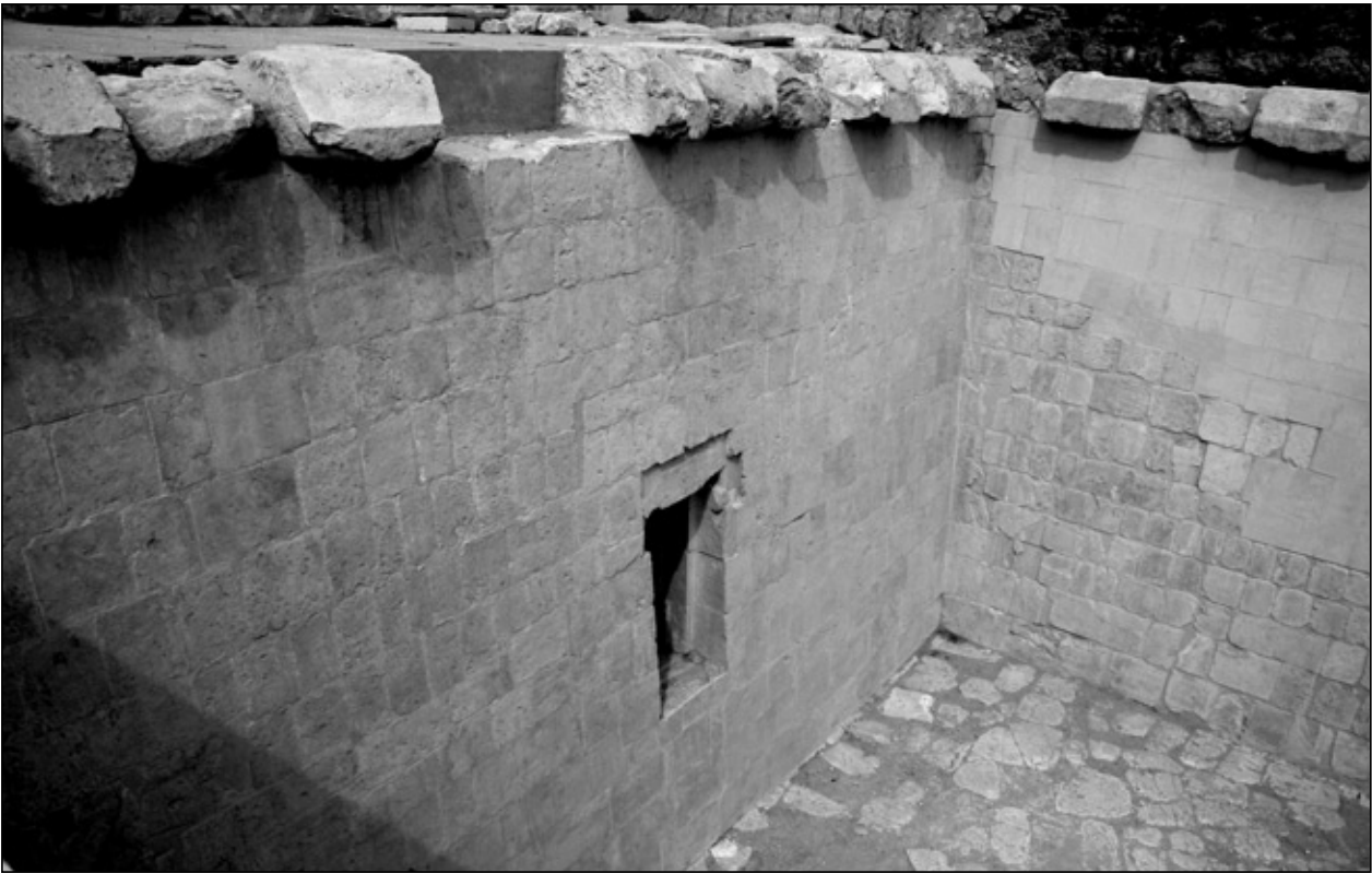
Fig. 2. Solar Cult Complex, North Wall. Blocks of the cornice after restoration (Photo M. Jawornicki)
