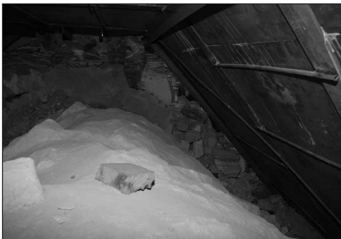
Fig. 4. View of the protected vault following the present work (Photo M. Jawornicki)
