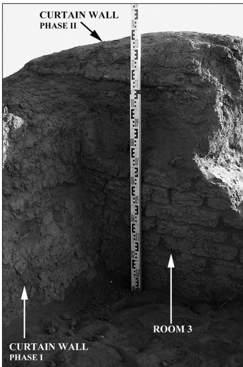
Fig. 10. Two phases of the curtain wall in Sector VII. February 2007 (Photo M. Drzewiecki)
