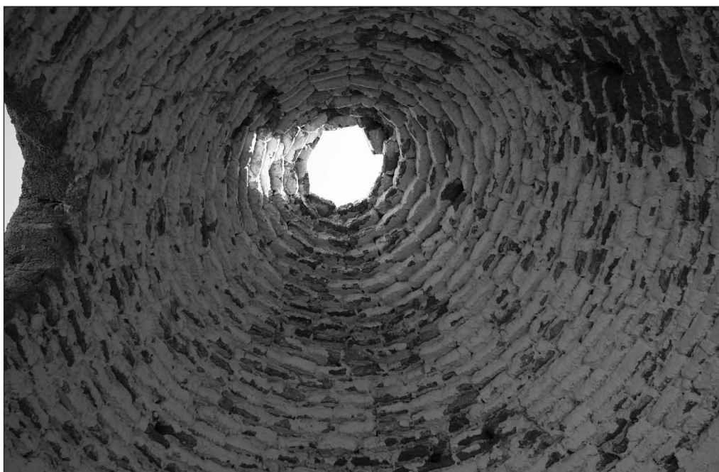
Fig. 6. Traditional qubba with cupola roof made of mud bricks and covered with plaster (top) and example of mud brick usage in cupola roof construction, both from Qaramel village (Photos R.F. Mazurowski)
