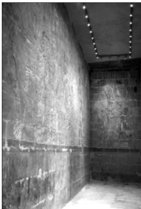
Fig. 6. Interior of the Northern Chamber of Amun-Re after restoration (Photo M. Jawornicki)
