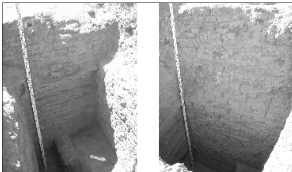
Fig. 10. Trench VII/2, outer face of wall II (right) and remains of structures erected against the outer face of this wall
