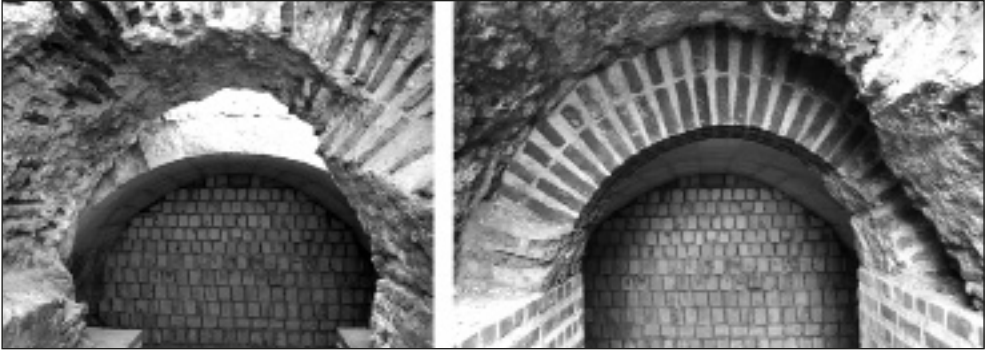
Fig. 13. One of the restored vaults giving access to the furnaces in the baths, before (left) and after restoration (Photo A. Pisarzewski)
