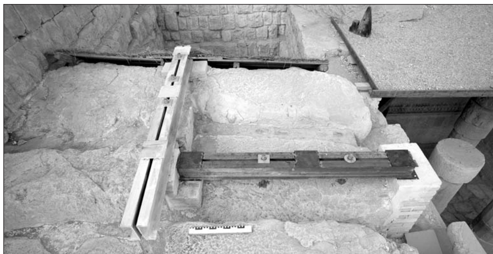
Fig. 8. Roof of the Harbor Shrine vestibule reinforced with a steel construction (Photo W. Wojciechowski)
