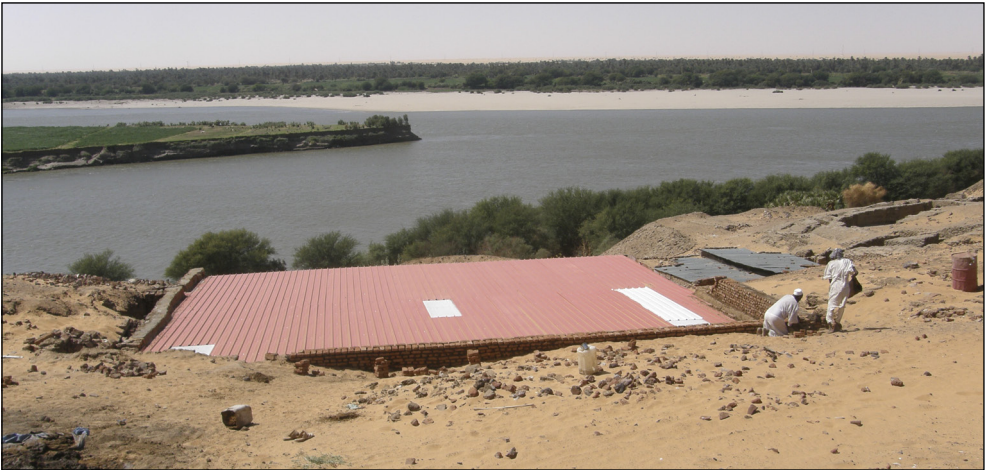
Fig. 6. View of the shelter constructed over the central and eastern parts of building B.V (Photo W. Godlewski, PCMA archives)
