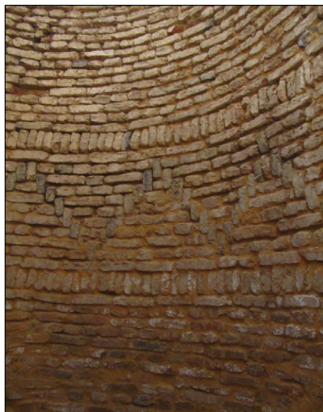
Fig. 9. Interior of the well ( matara ) at Selib with zigzag pattern of bricks in the lower part (Photo A. Cedro)
